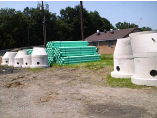
Construction begins on the Factoryville Borough/Clinton Township Joint Municipal Authority wastewater improvement project.
